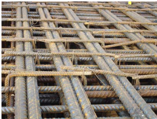
A typical situation in the field - not according to building standards.
